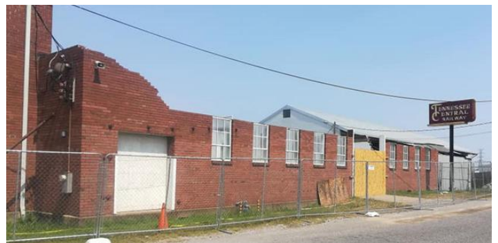
Lest we forget where we were - Demolition- Roof Trusses and Bricks Above Windows Removed - Photo by Jason Sharpe -
