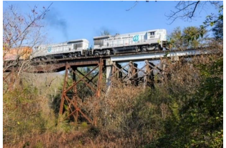
Timezone/ Piney Creek bridge from the highway - Photo by Sam McAllister. Note the steel piers in the middle and wooden ones towards the abutment.
