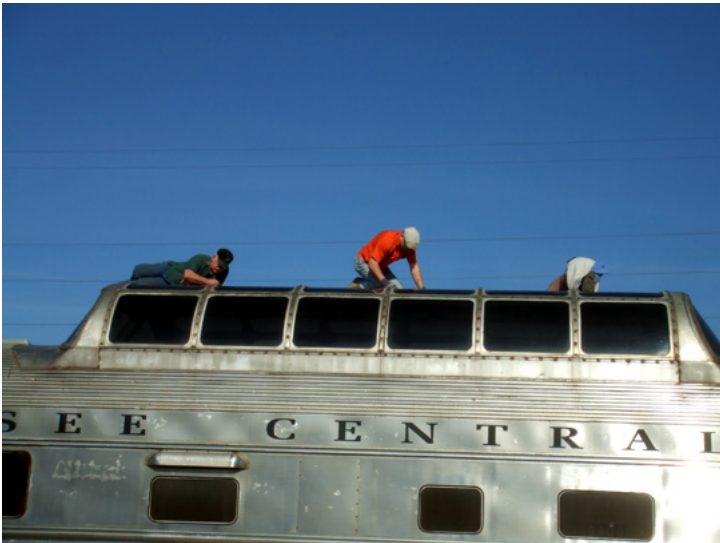
TCRM members working on the dome of TCRX 9400. This car has some leaks we are trying to stop. Photo by Terry Bebout
